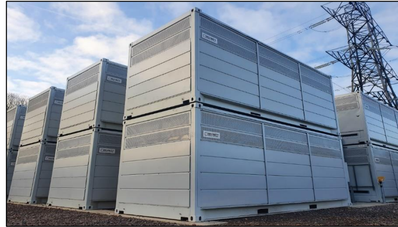
Vanadium Flow Batteries installed at Oxford Superhub
